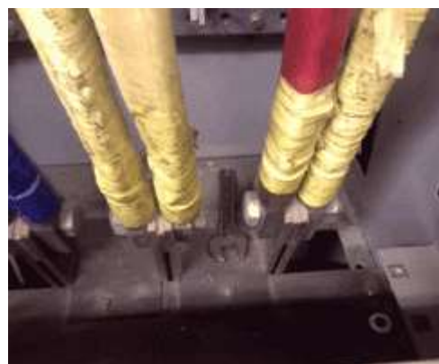
Part of the video used for the Duty Holder (Authorised Person) course, depicting some of the issues surrounding live working
